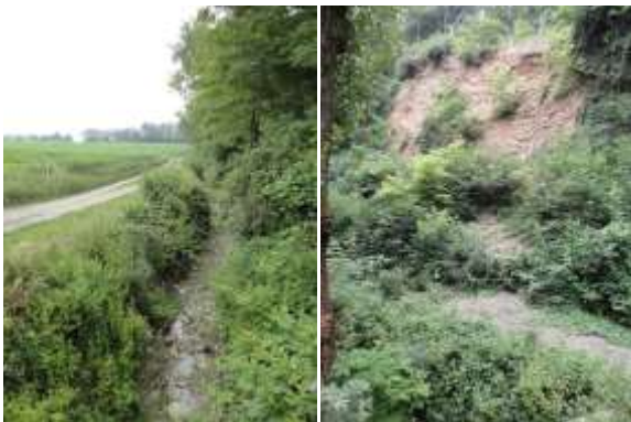
Left: the local roads directly affects the streambed of the Rio Lavezza creek; right: stretch erosion on Rio Enzola creek
